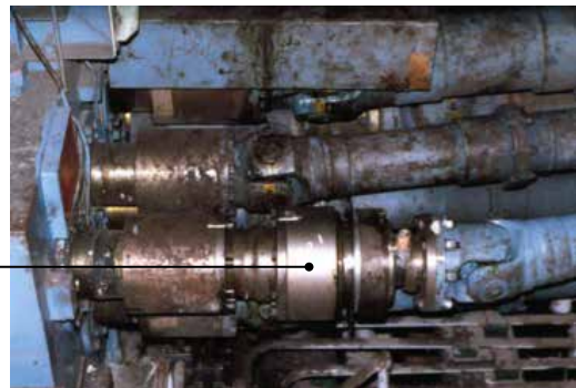
Pictured above: A special Autogard Torque Limiter installed on the output side of the drive. Torque limiters such as the Autogard 820 Series are generally installed on the input side of the drive for overload protection.
