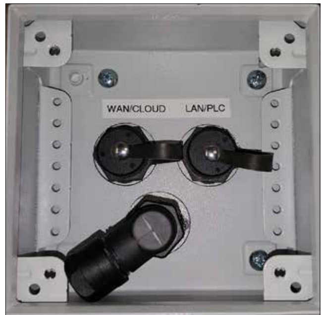
Figure 2 – AC Power and Data Connections inside interface box
