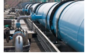
Electric water pumps
