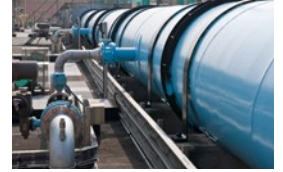
Electric water pumps
