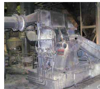
Large fan at cement plant in Indiana moves air through a rotary kiln. Bearing failures from vibration and contamination led to replacing them with Rex 6000 SHURLOK Adapter Mounted Roller Bearings.
