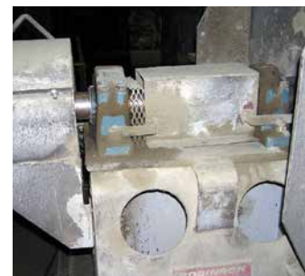
Previous bearing was a split housing that had to be assembled onsite, allowing cement dust to contaminate the lubricant. Its lock nut would loosen because of fan-induced vibration, leading to premature failure.
