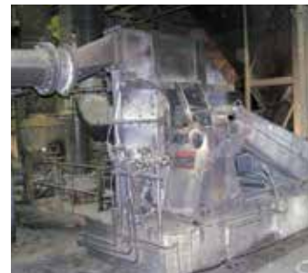
Large fan at cement plant in Indiana moves air through a rotary kiln. Bearing failures from vibration and contamination led to replacing them with Rex 6000 SHURLOK Adapter Mounted Roller Bearings.
