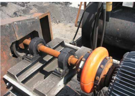
Closeup shows two Rexnord Bearings supporting jackshaft and Omega Coupling connecting motor to shaft.
