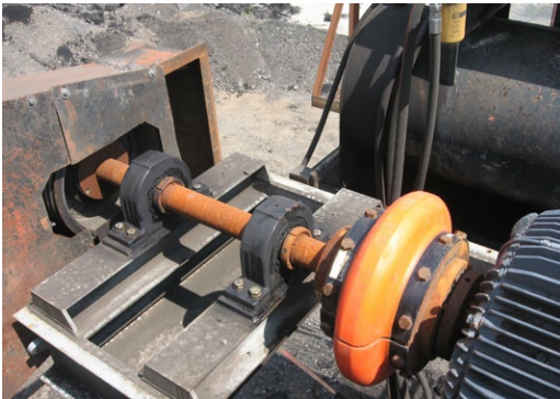
Closeup shows two Rexnord Bearings supporting jackshaft and Omega Coupling connecting motor to shaft.
