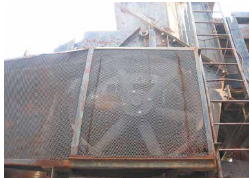
View from opposite side shows large multiple V-groove pulley that drives the crusher (inside guard).
