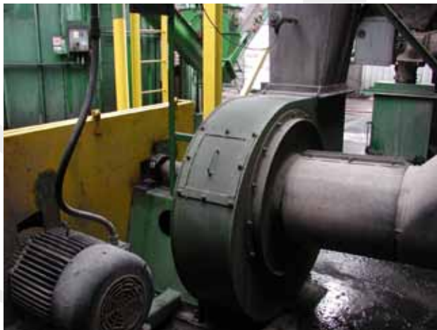
Bearings on this induced draft fan at a major hardwood mill were failing frequently before they were changed to Rexnord ZAF6000 Series SHURLOK® Adapter Mounted Roller Bearings.
