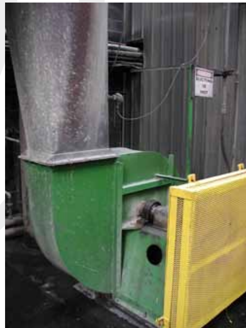
Closeup shows new bearings in place, with induced draft fan housing at right and guard for V-belt speed increaser at left.
