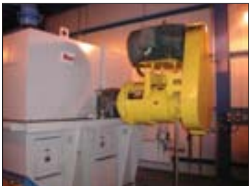
Titan with 36:56:1 ration driven by 100 HP motor on a Rexnord High Load Elevator.
