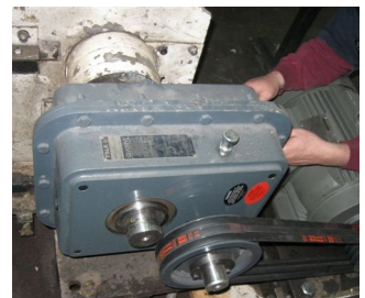
A Falk Quadrive with the proper service factor was installed, delivering 94% savings per year.
